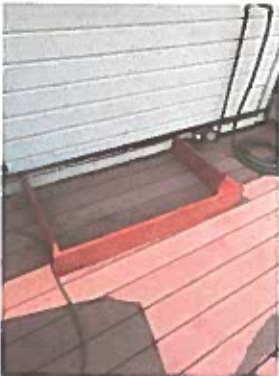
D) Picture of wood brace to keep LPG Grill 2 feet from home.
