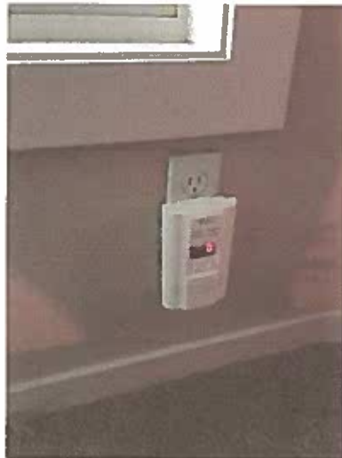
C) 2 Additional LPG Detectors by water heater and on main level of the home.
