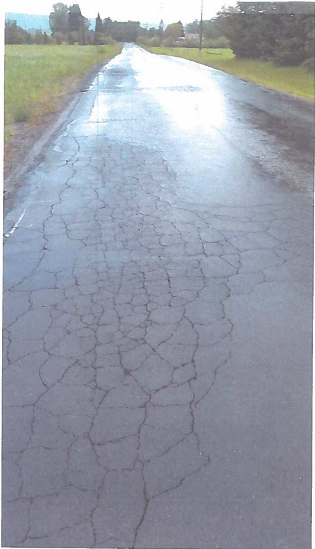
Photo 3: Another area of deterioration of Pearson Lane at site, looking west.
