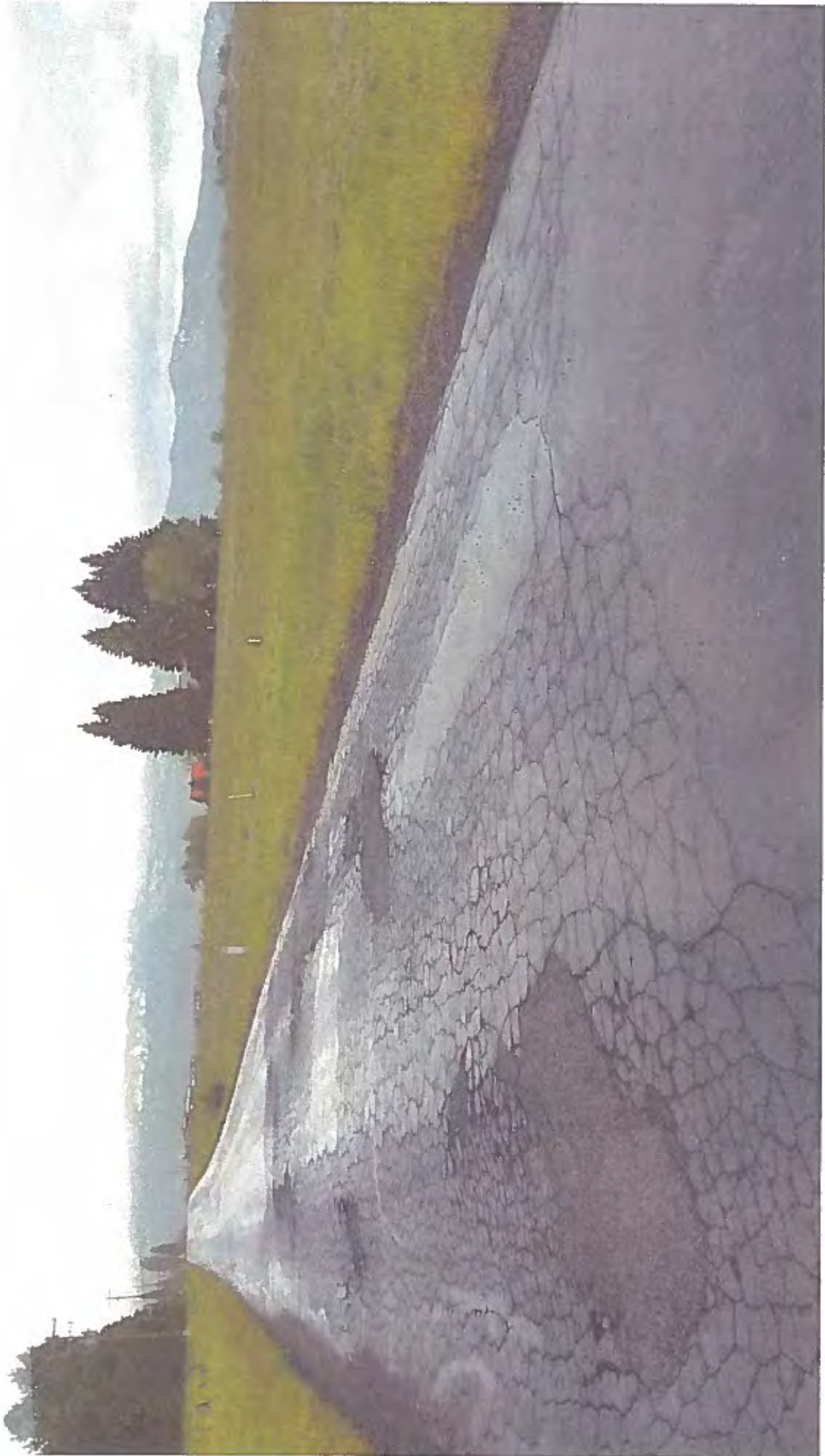
Photo 2: Condition of Pearson Lane where access driveway planned, looking east.
