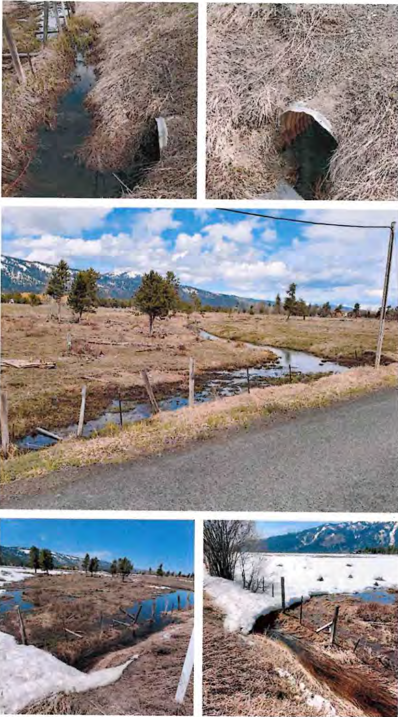
Figure 2, Wendell Platt Property @ Norwood Rd culvert down gradient of project: Top & mid views May 2, 2022 and bottom snow-covered views May 3, 2023. The ditch and pipe covered in snow freeze in the winter and back up flow during fast spring thaws. The concern is that this partially sediment filled pipe will not be able to handle the new hydraulic loading of multiple new upgradient developments.
