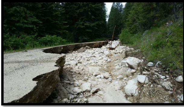
Washout on Lick Creek RD
