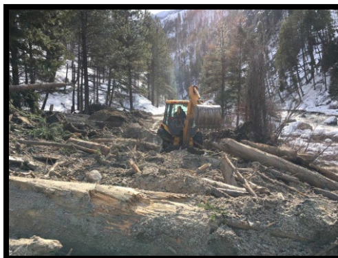
Landslide on East Fork Road
