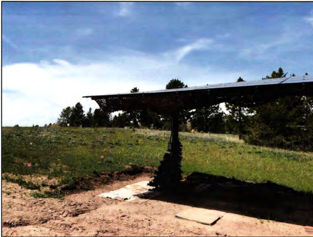
Photo 10. View looking north/northwest at solar array directly north of garage. The camouflage netting was not intended to be a permanent solution for screening. Photo: Mark McClellen 5/10/2026
