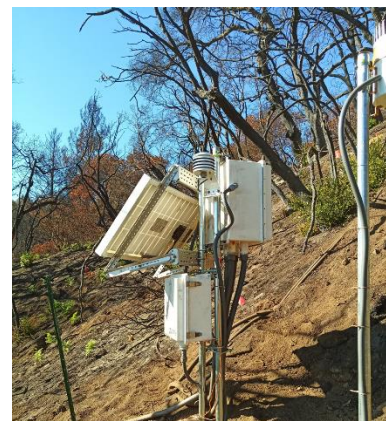
USGS rainfall/soil moisture gage that was recently installed for the CZU burn scar above Boulder Creek. Ownership of the equipment will transfer to the County following initial technical support and maintenance
