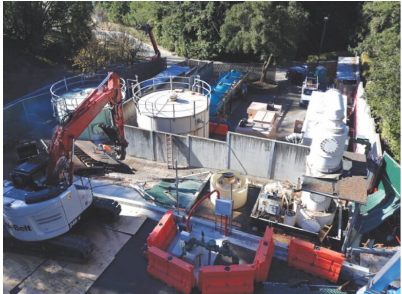
Orchard Run Treatment Plant Project began demolition in December and should be completed by May 1
