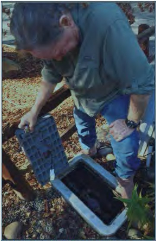
Ekwall simultaneously reveals the i-Meter at his home and the site of a leak.
