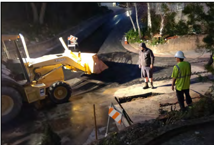
The crew worked until about 9 pm to secure the site and clean up. Here the crew is using a loader to maneuver two steel plates into position over the hole.
