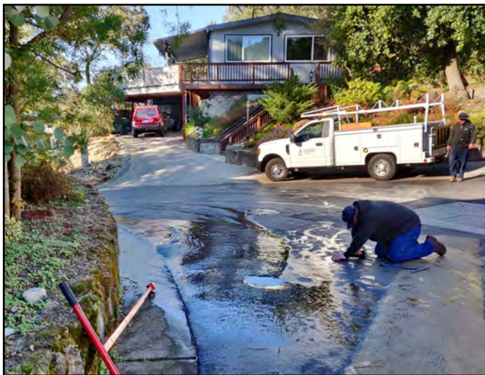
A worker from SV Water District checks a water main valve.
