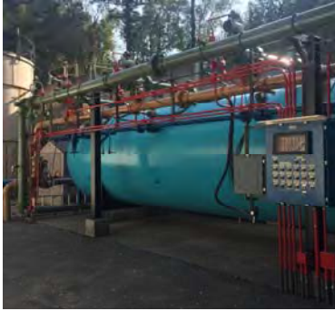
Orchard Run Water TP (1993) 1.3 million gallons per day (MGD) $3M+ for improvements Construction to commence Dec 2020
