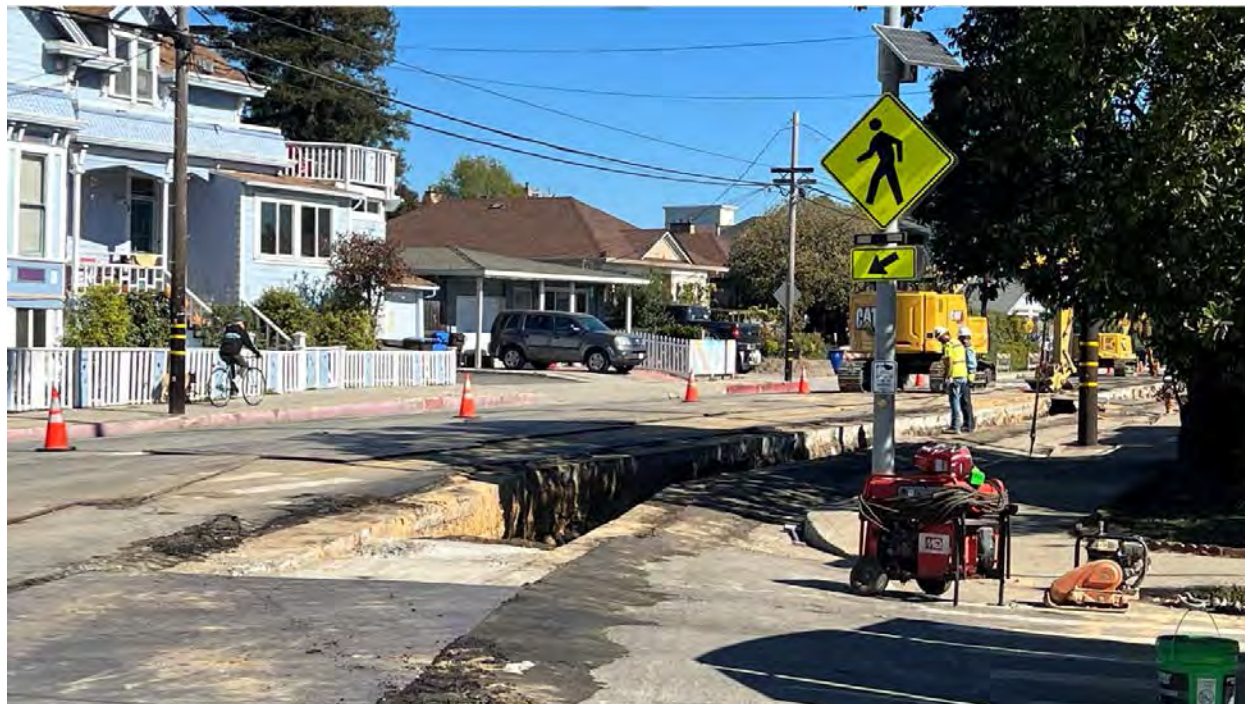
Workers install a water pipe on Broadway from Riverside Avenue to Clay Street in Santa Cruz in February as part of the Pure Water Soquel Conveyance Project. (Brian Phan — Santa Cruz Local)
